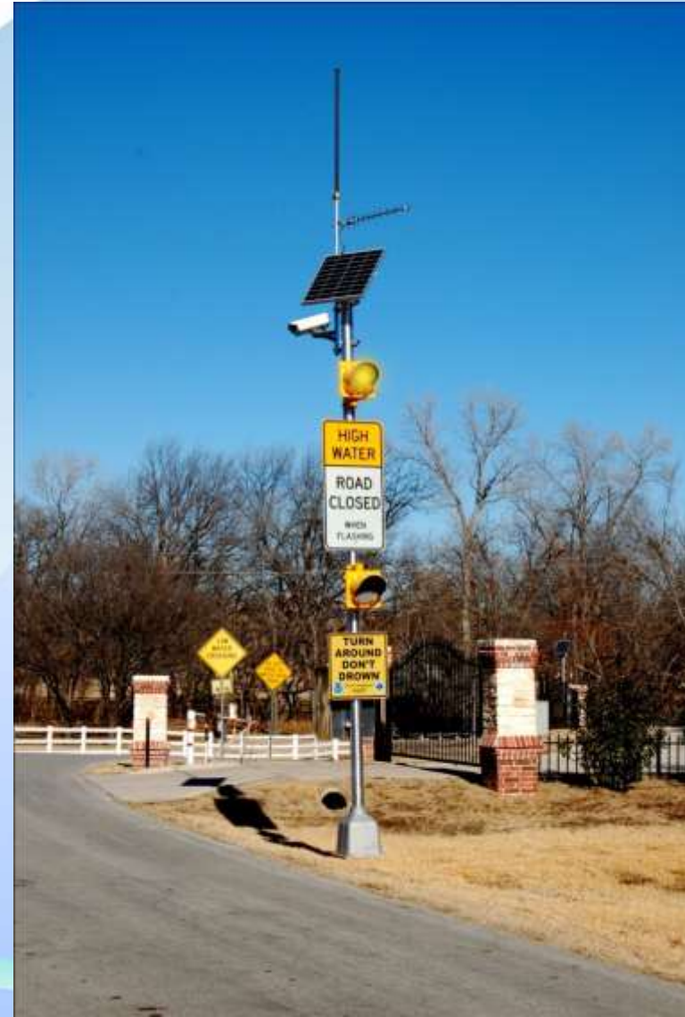
Flooded Roadway Warning System with on-demand video monitoring City of Colleyville, TX
