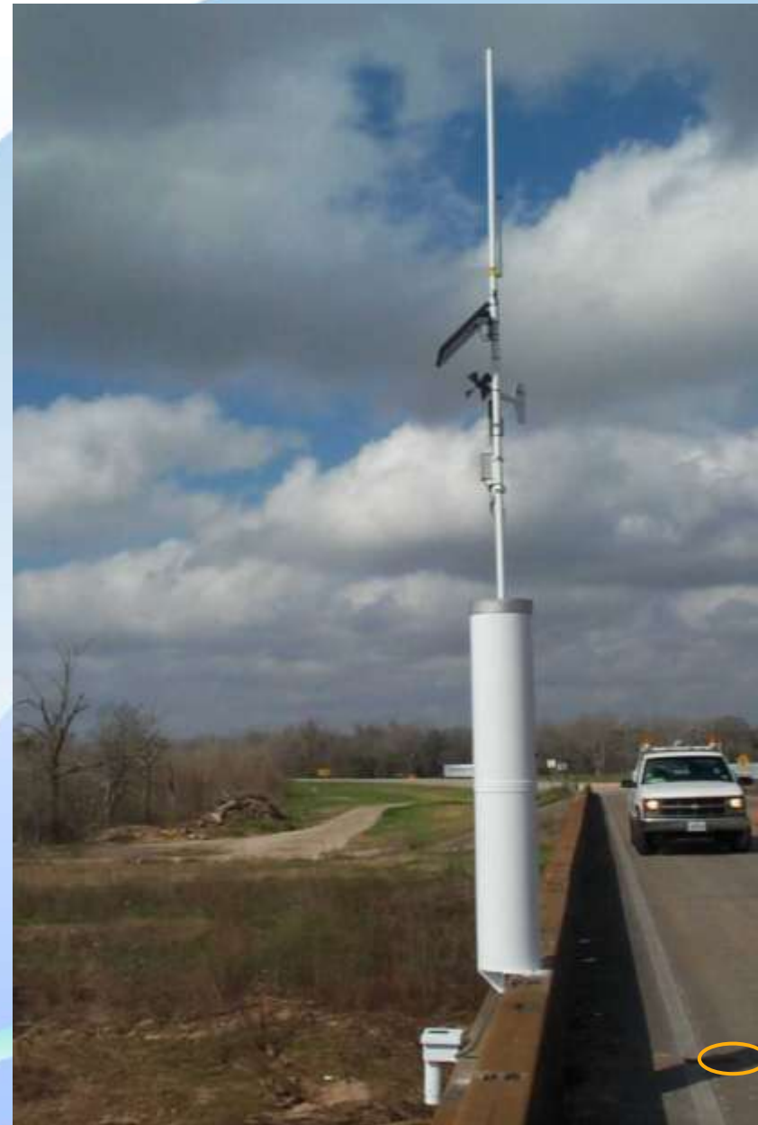
TxDOT Bridge Mount Weather & Stream Monitoring System SH35 at Brazos River
