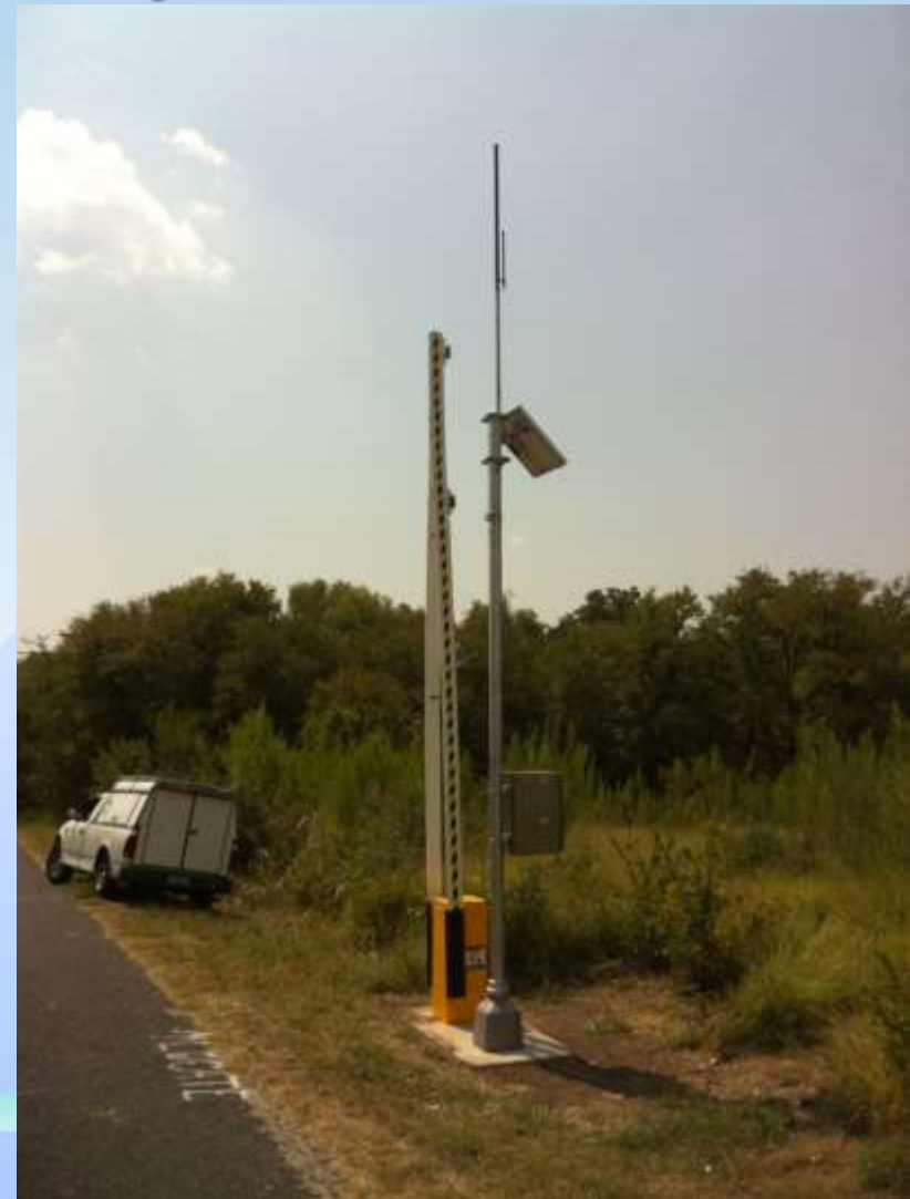
Flooded Roadway Warning System with Automatic Barrier Gates W.W. White Rd, San Antonio, TX
